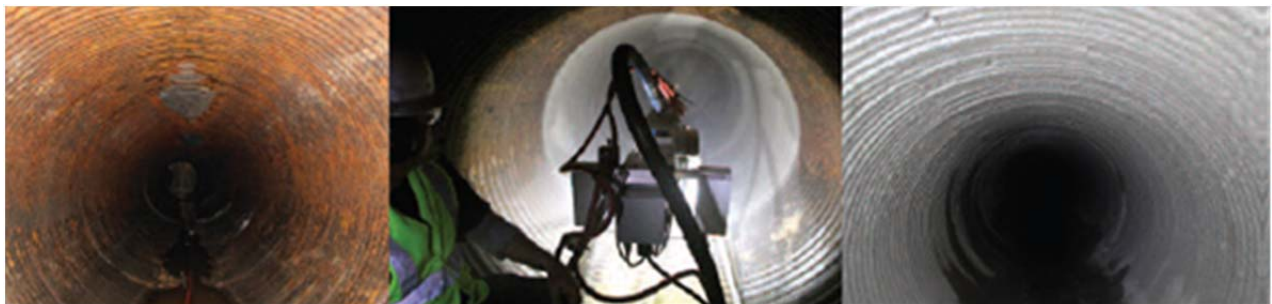
Figure 2: From left to right (a) Leaking storm water culvert (b) Centrifugal application of GeoSpray™ (c) Completed Repair 11
